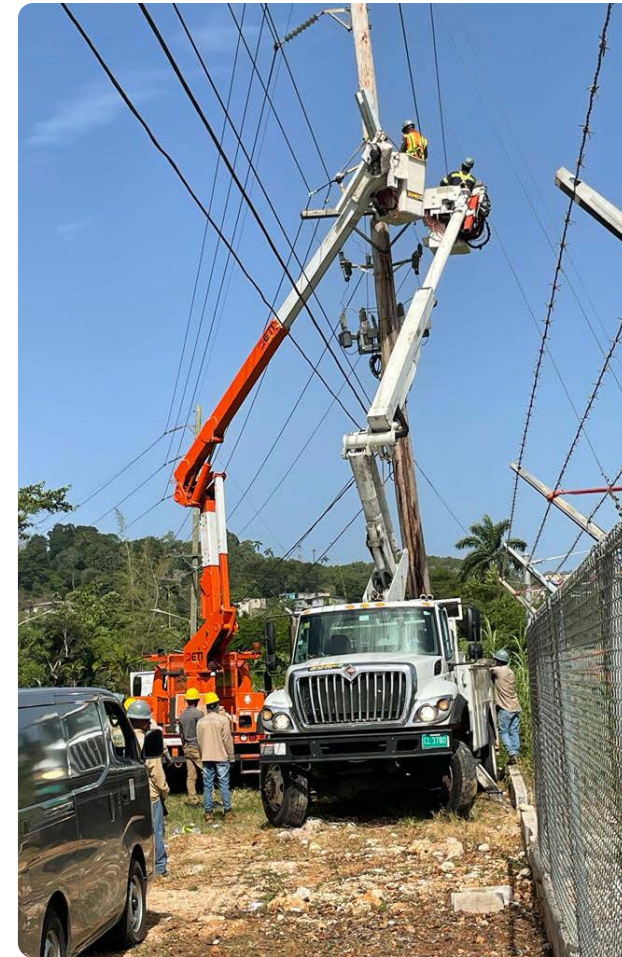
SYSTEM MAINTENANCE: Members of the Manchester Operations team installing cross arms during routine maintenance work.
