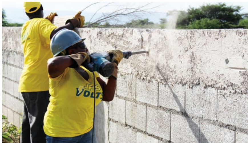
Members of the JPS' volunteer arm VOLTS (Volunteers On Location To Serve), get busy working on the perimeter wall for the York Town Basic School.
