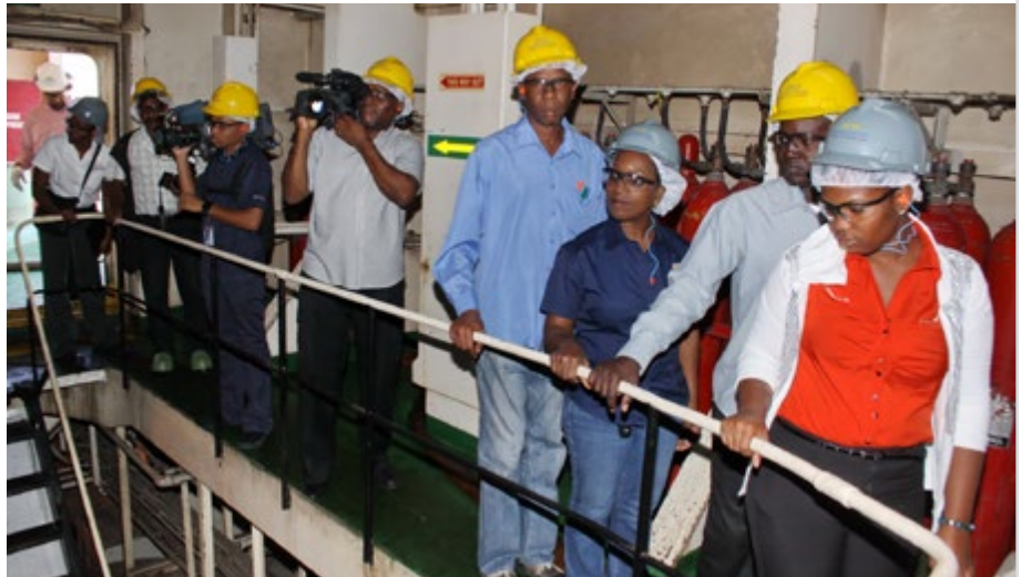
Members of the media are guided on a tour of the Rockfort Power Plant in East Kingston, as Unit 2 of that facility undergoes major overhauling to improve efficiency.
